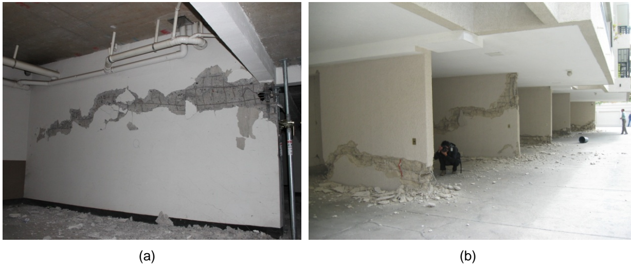
Figure 2-1 Typical reinforced concrete shear wall damage in the 2010 Maule earthquake: (a) first subterranean level of an 18-story building in Santiago (photo courtesy of Jack Moehle); and (b) ground floor level of a 10-story building in Viña del Mar (photo courtesy of Patricio Bonelli).
