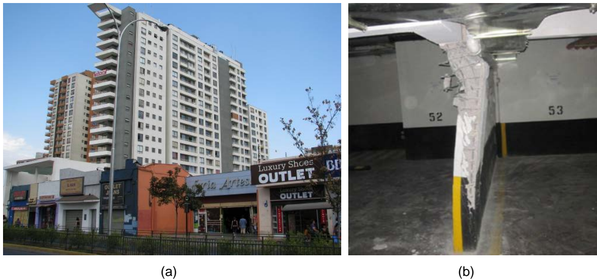
Figure 3-9 Undisclosed Building B: (a) exterior elevations; and (b) wall buckling in the first subterranean level along transverse Line O (DICTUC, 2010e).
