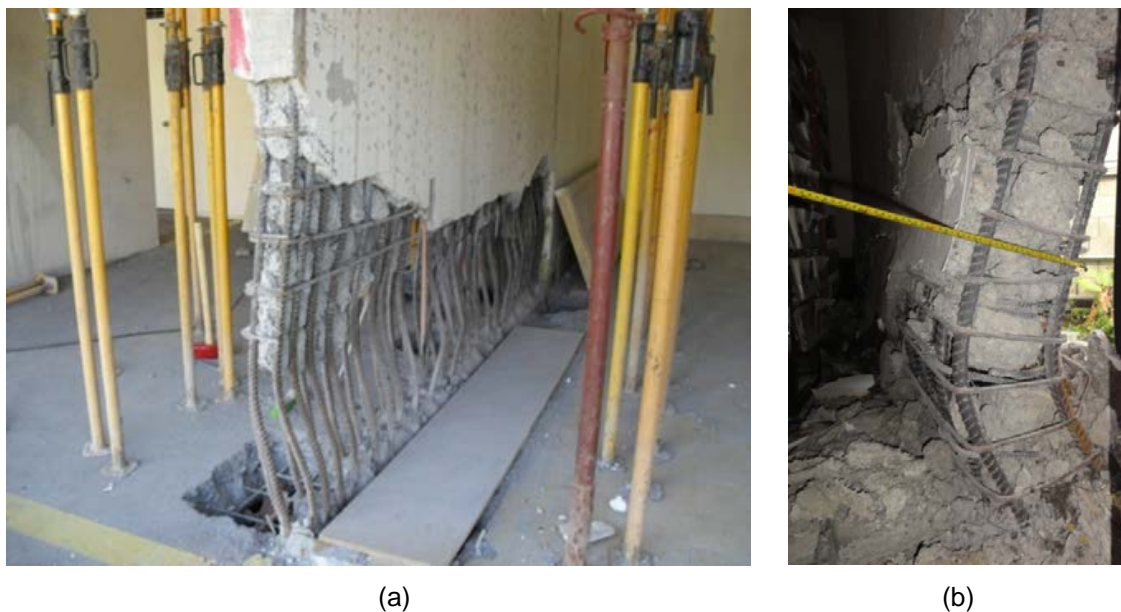
Figure B-1 Examples of wall lateral buckling: (a) 2010 Maule earthquake (DICTUC, 2010d); and (b) 2011 Christchurch earthquake (photo courtesy of Ken Elwood).
