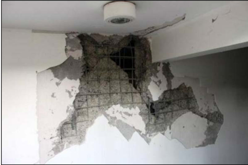
Figure 4-17 Damage observed in a solid wall panel below a stack of openings in the Torre Mayor building, Chillán (photo courtesy of EERI).
