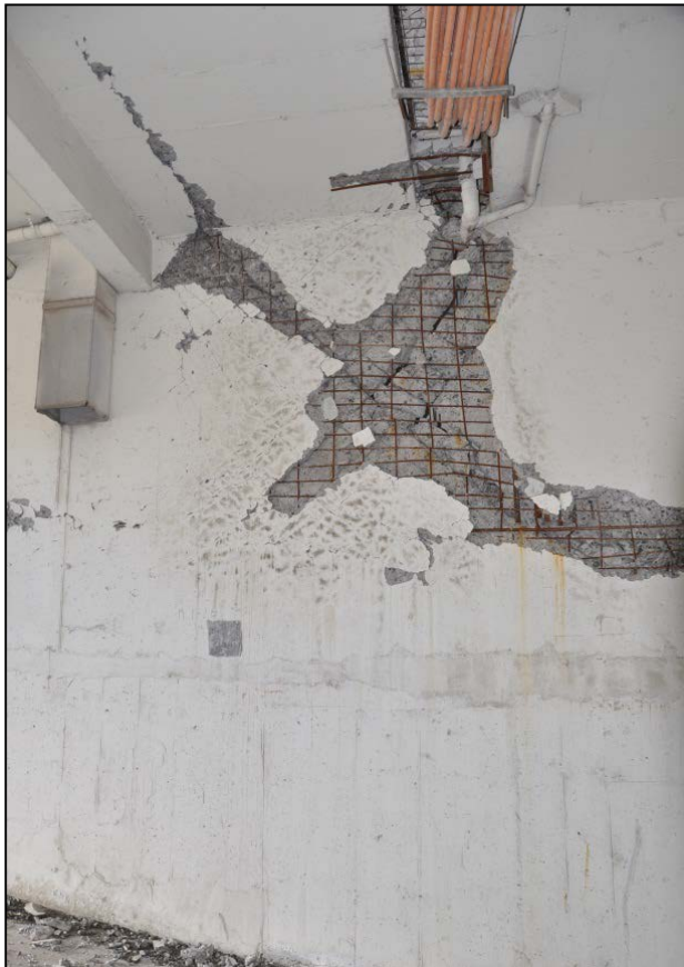
Figure C-4 Damage observed in solid panel at the bottom of a stack of openings in the Centro Mayor building in Concepción, Chile following the 2010 Maule earthquake (photo courtesy of EERI Chile earthquake reconnaissance team).
