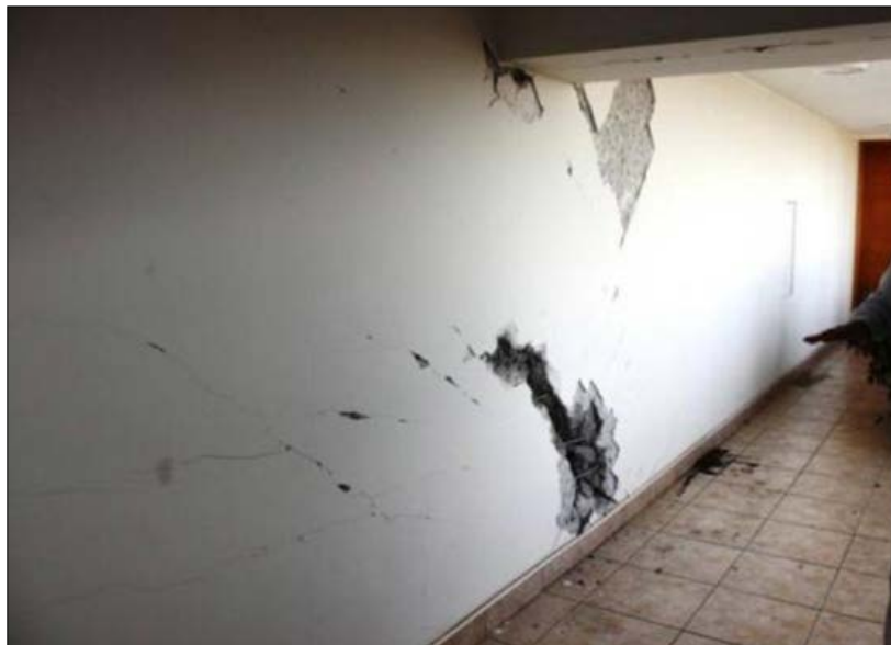
Figure 4-16 Damage observed in a solid wall panel above a stack of openings in the Torre Mayor building, Chillán (photo courtesy of EERI).
