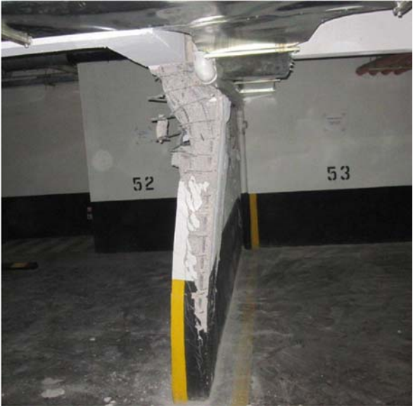
Figure 1-7 Overall wall buckling behavior (DICTUC, 2010e).
