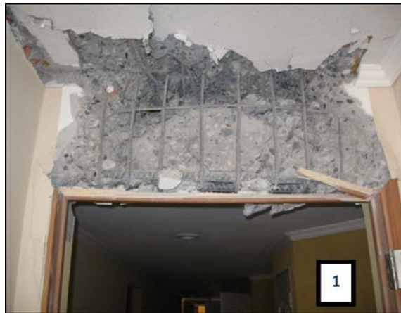
Figure 4-31 Damage to coupling beam in the Centro Mayor building, Concepción (DICTUC, 2010b).
