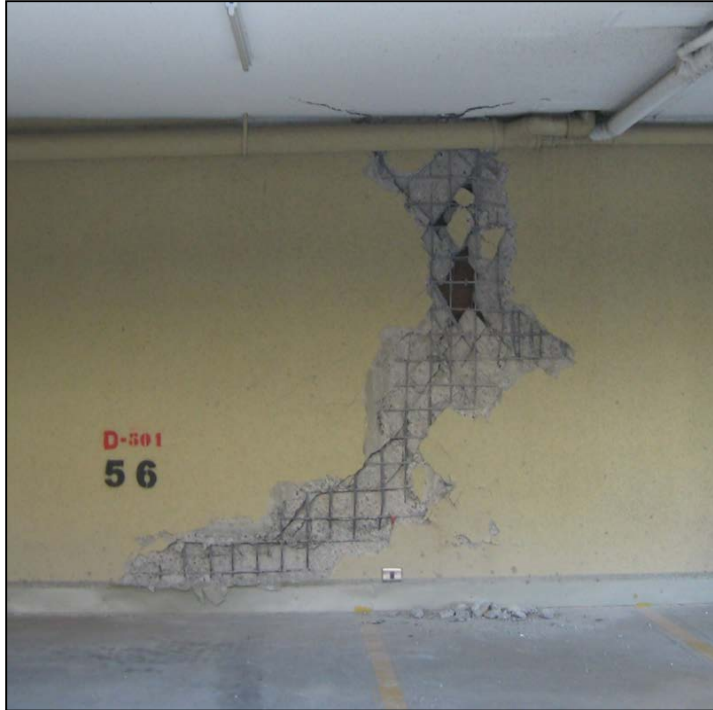
Figure C-5 Damage observed in solid panel at the bottom of a stack of openings in the Marina del Sol building in Viña del Mar, Chile following the 2010 Maule earthquake (photo courtesy of Patricio Bonelli).
