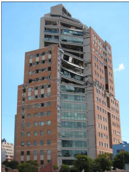
Figure 4-13 Photograph of damage to the O'Higgins building, Concepción. Damage was attributed, in part, to vertical discontinuities in the building configuration. Significant damage, including partial collapse of upper floors, was observed (photo courtesy of Joseph Maffei).
