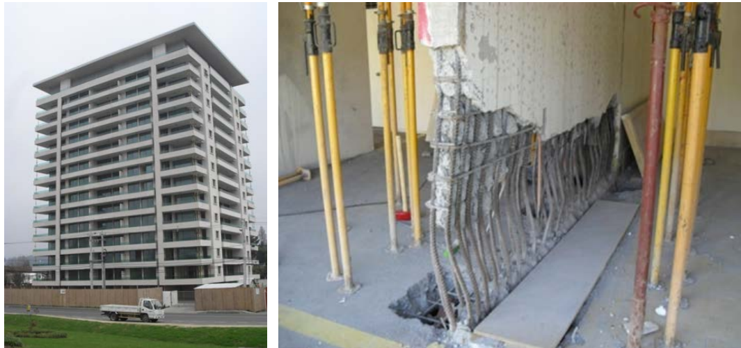
(a) (b) Figure 3-4 Alto Huerto building: (a) East elevation; and (b) wall crushing and apparent wall buckling along Line Ñ (DICTUC, 2010d).
